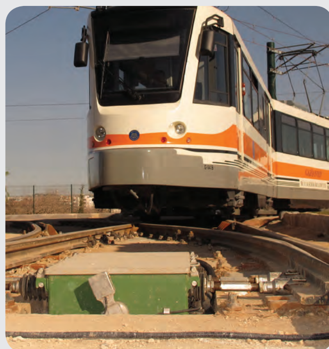
Complete system including Elektroline point machines
