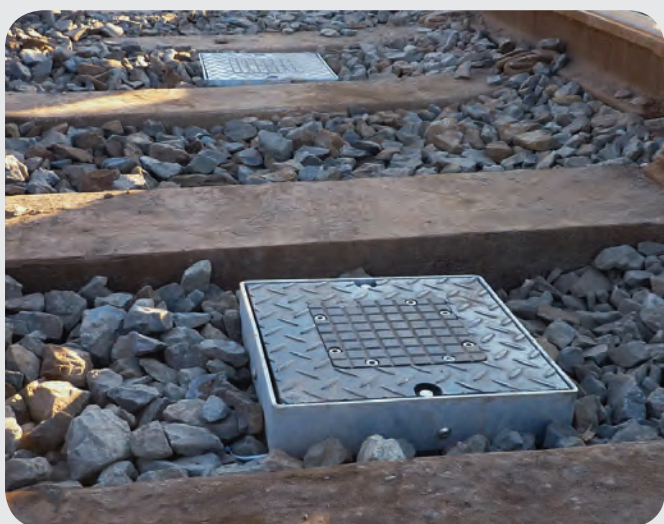
Ground VETRA transponder installed in track
